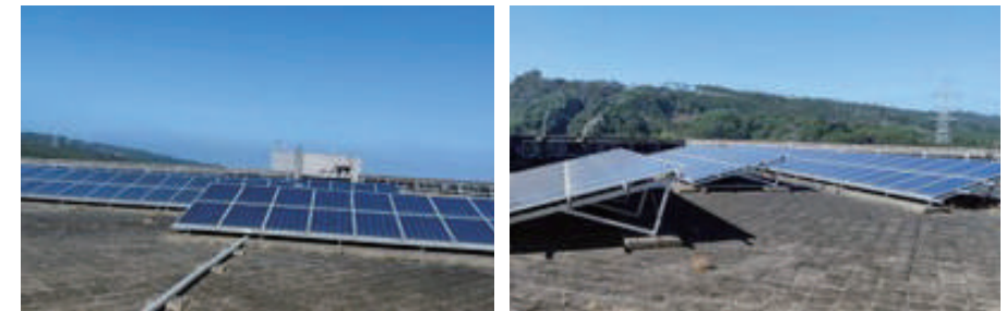
PV power generation system of Nankang Plant
